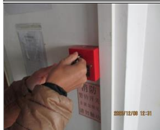
Photo of fire safety equipment Alarm testing.JPG
