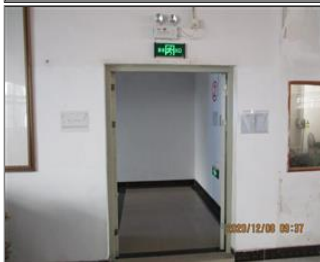
Photo of fire safety equipment Emergency exit with sign.JPG
