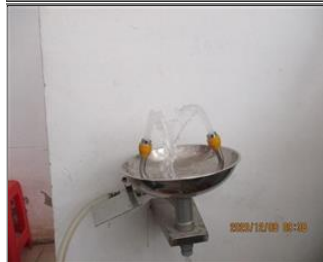
Photo first aid facilities Eye washing facility.JPG
