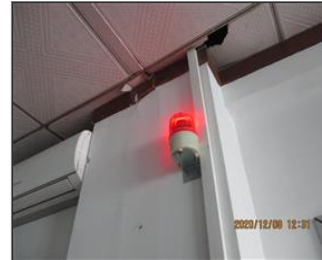
Photo of fire safety equipment Visual alarm testing.JPG
