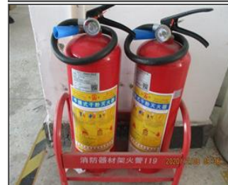
Photo of fire safety equipment Fire extinguishers.JPG
