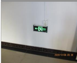
Photo of fire safety equipment Evacuation sign.JPG
