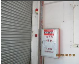
Photo of fire safety equipment Hydrant.JPG
