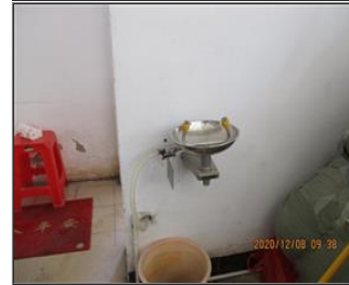
Photo of non-conformity NC-No eye washing guideline nearby eye washing facility.JPG
